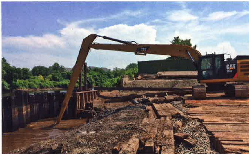
Boswell Engineering is in the midst of cleaning the former River Oil Terminal in Passaic - for which the LSRP process will decrease the timeframe of the previous NJDEP review and approval process by about three years.
